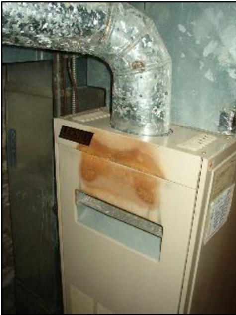
Draft hood spillage or backdraft
