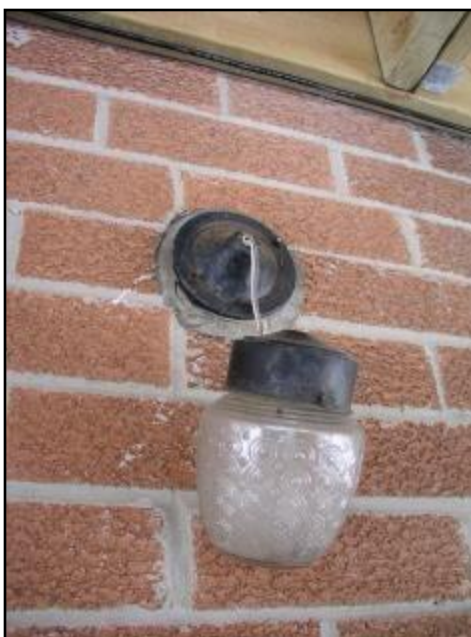
Light fixture is not well secured
