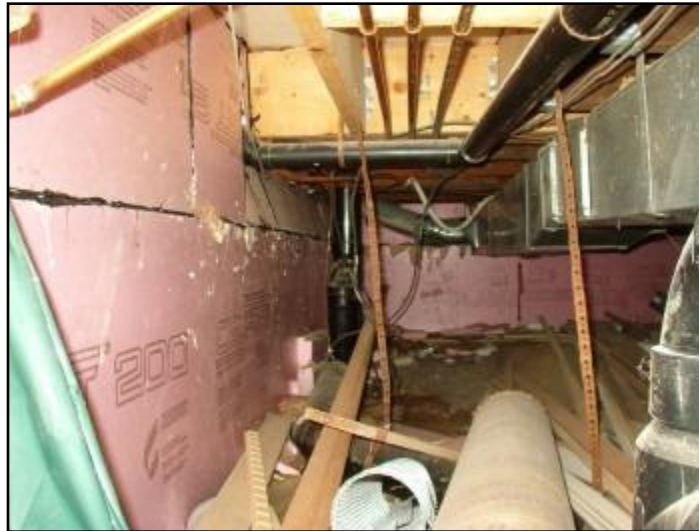
Exposed combustible insulation
