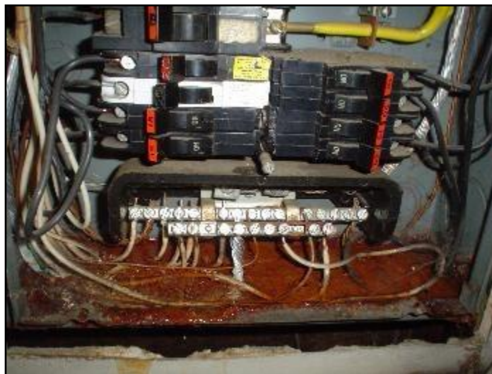
Water and rust in bottom of panel
