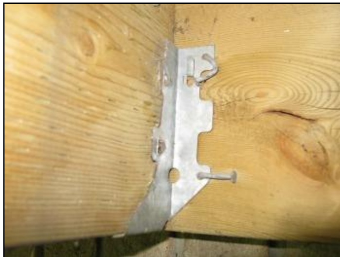
Poor end bearing, joist hanger connections
