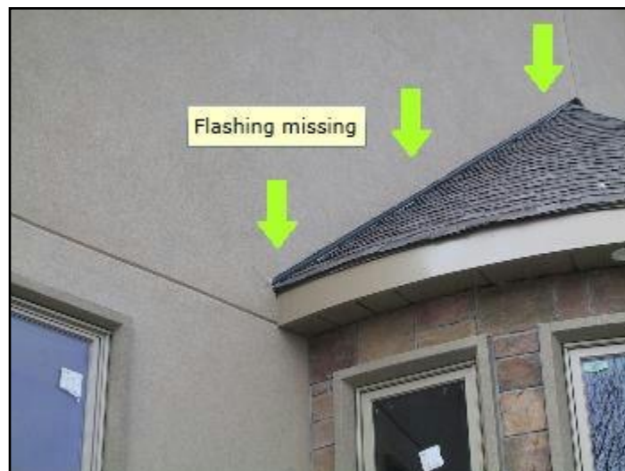
No kickout flashing at roof/sidewall junction
