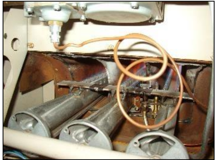
Draft hood spillage or backdraft
