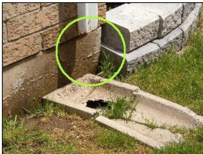
Downspouts discharge too close to building
