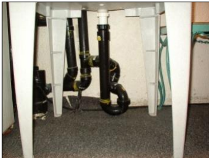
Poor trap arrangement
