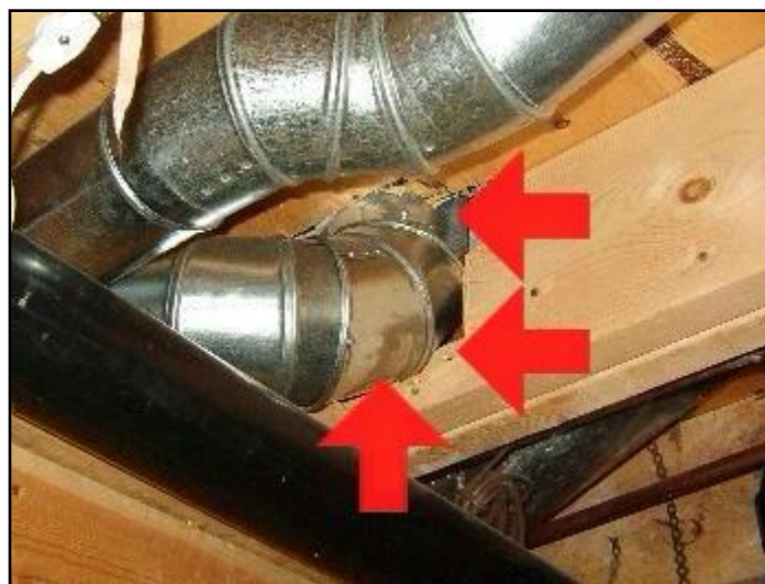
Joists are notched and weakened
