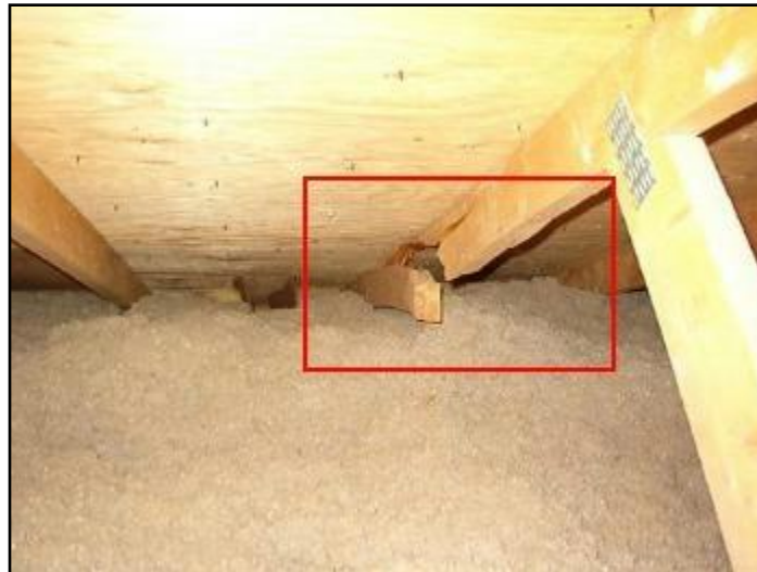
Top chord of truss is split
