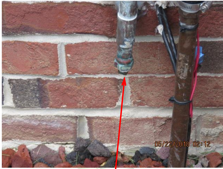
Leak at sprinkler
