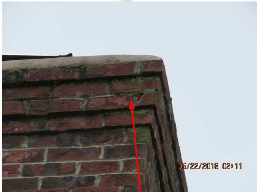
Spalling brick on chimney
