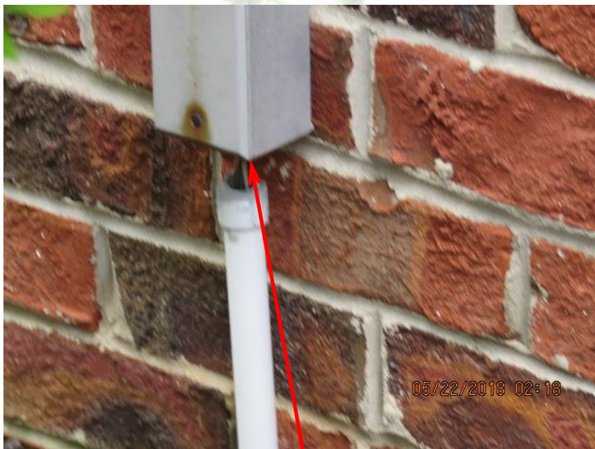
Wiring separated from junction box
