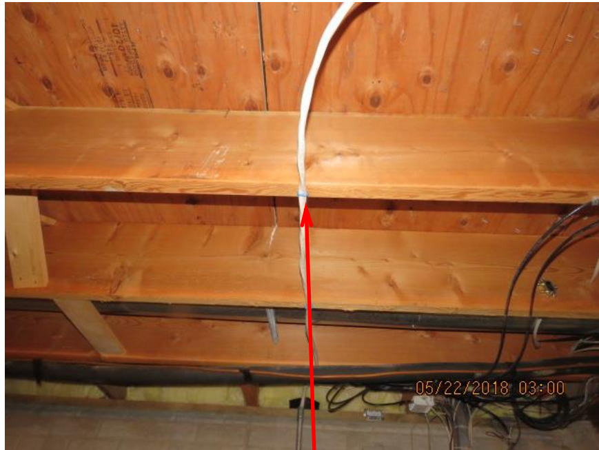
Exposed nonmetallic wiring
